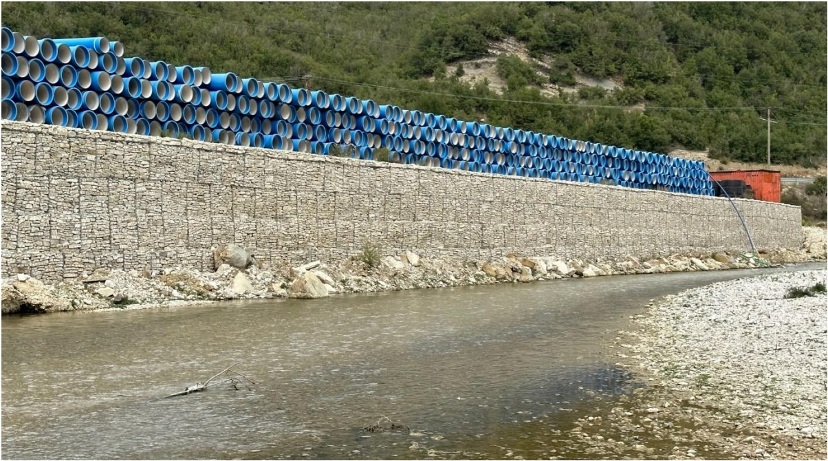
Figure 20: Construction site for a water supply channel at the Shushica tributary (Picture: Riverwatch/Ulrich Eichelmann)
