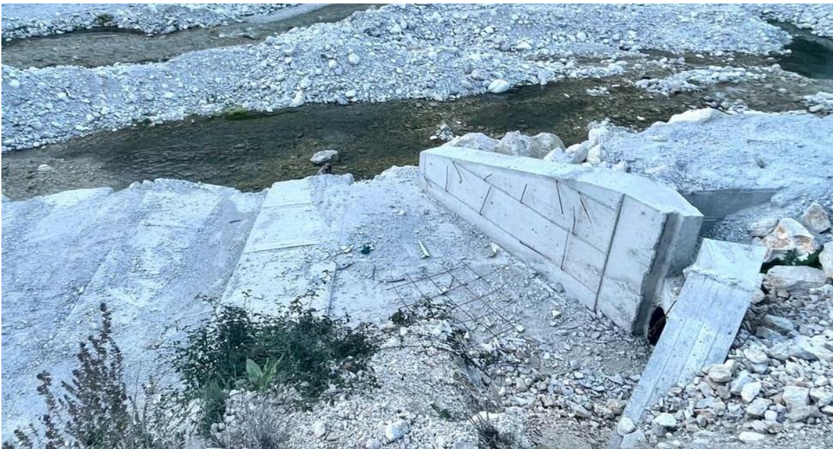
Figure 21: Construction of a new irrigation channel at the Kardiqi tributary (Picture: Riverwatch/Ulrich Eichelmann)
